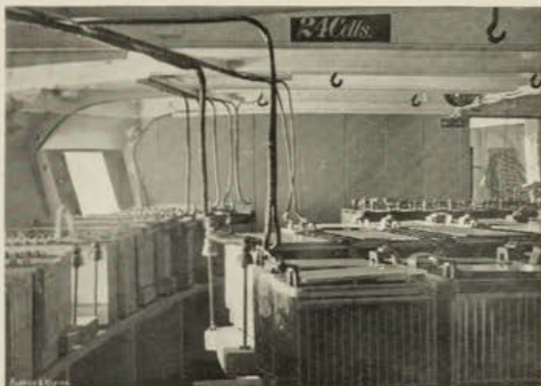
A PART OF THE SECONDARY BATTERY ROOM.
